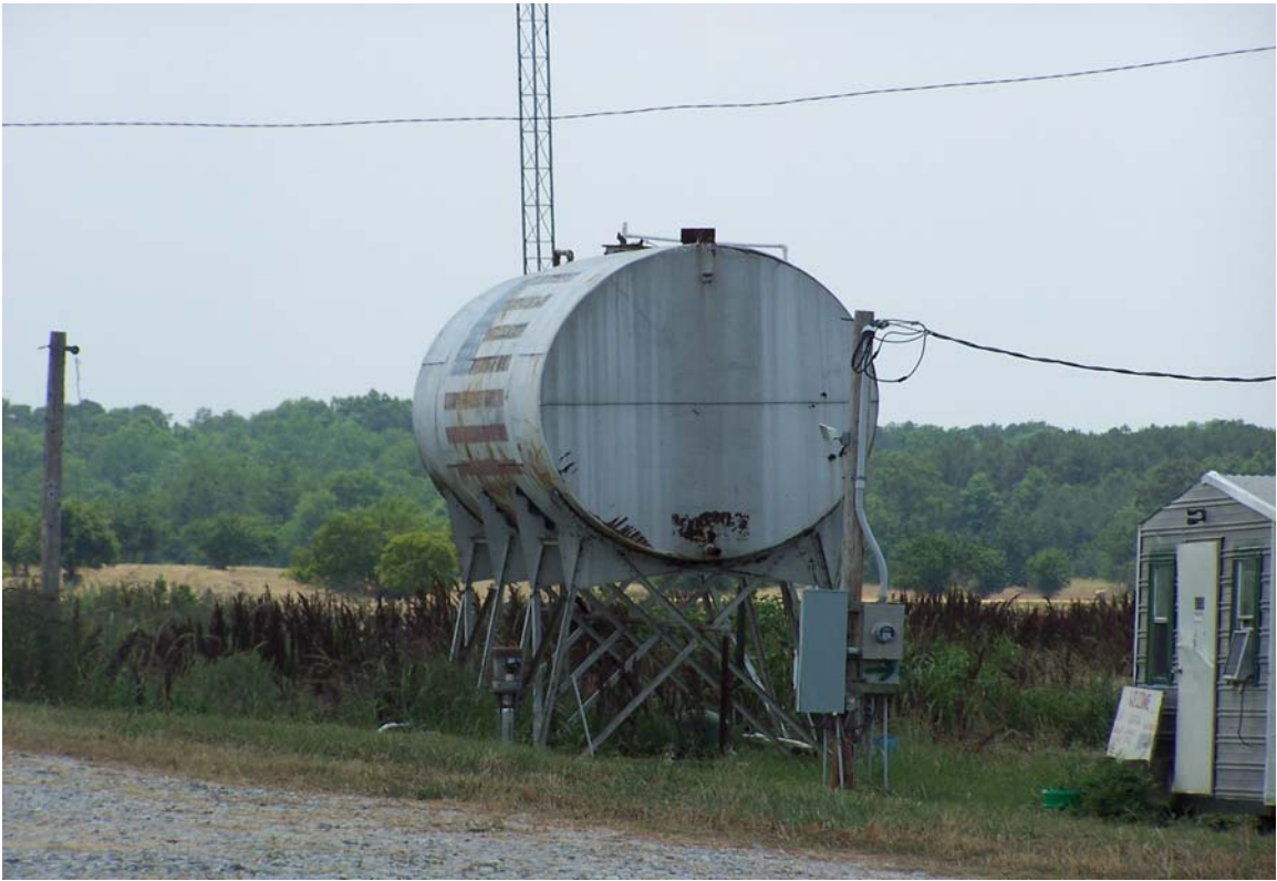
Photo 2: AST located at Scott's Trailer Wash
